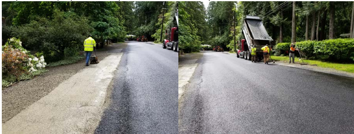
PSE adding shoulder material for a better walking surface to the recent overlay at NE 182St/40 th Ave NE.
