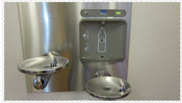
Lower Level Drinking Fountain
