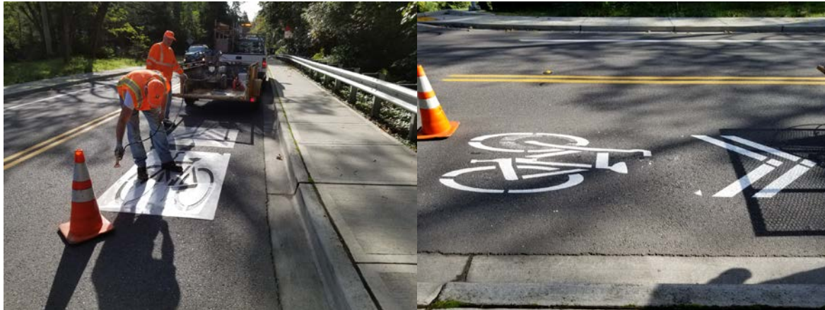
Traffic sharrows were repainted on NE 178 th St, Sept 25 by King County Traffic Division.
