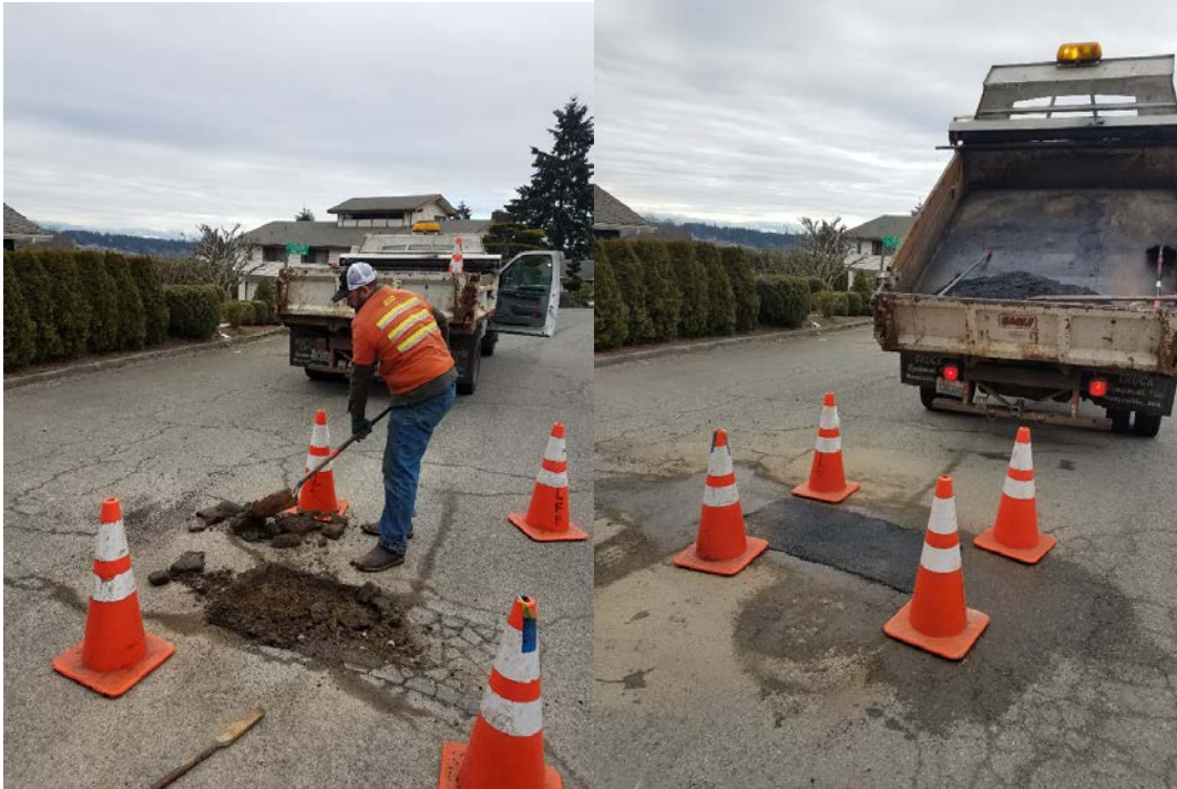
The repairs and work never slow down as the snow melts and the freezing temp begin to warm in the high 30's proactive pothole repair begins.
