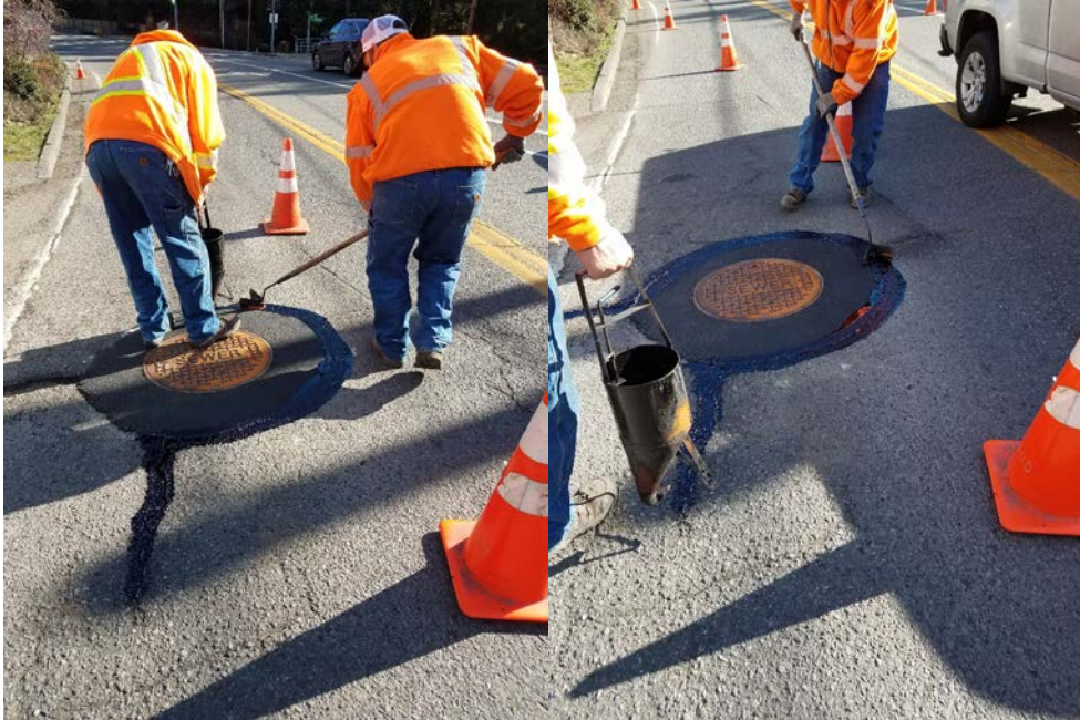
Repairing sanitary sewer manhole lid/frame @ SR-104 & 35 th Ave NE; the original lid had cracked and fell into the manhole. A Public Works crew member noticed the open manhole while driving and immediately stopped and conducted traffic control so no vehicle would drive into the open manhole and notified a supervisor. Repairs made Feb 26 th .
