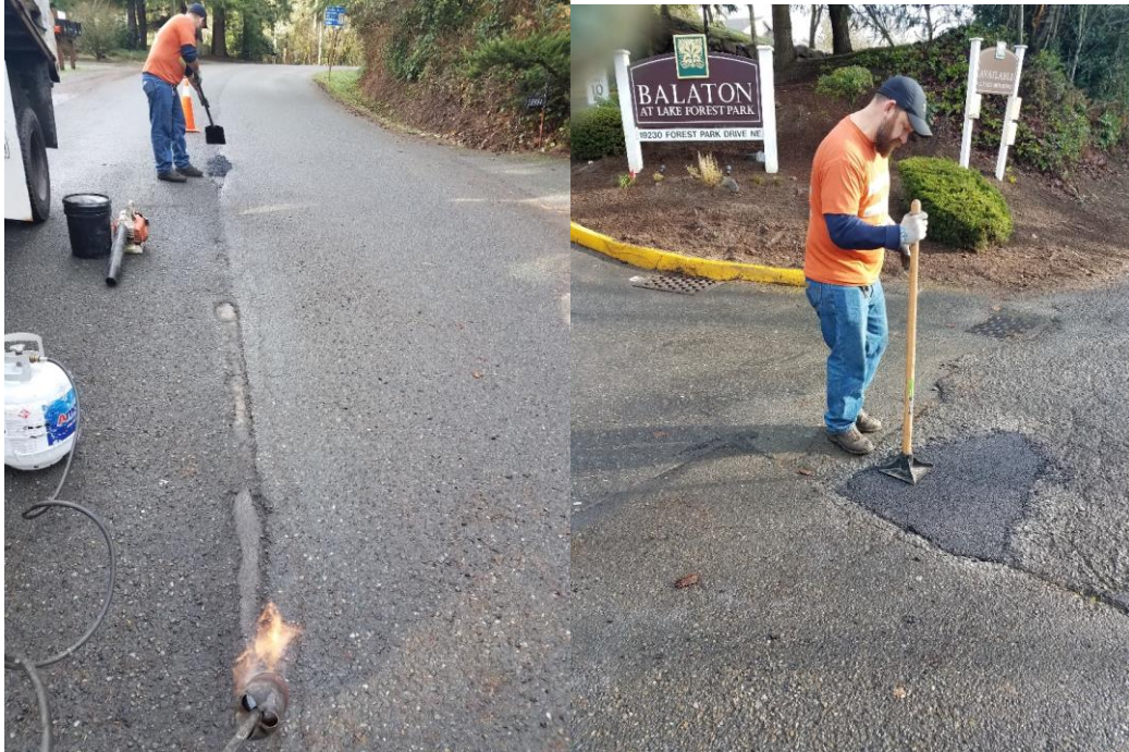
Public Works conducting pavement repair on Forest Park DR NE using a torch down method due to the slight dampness on the pavement.
