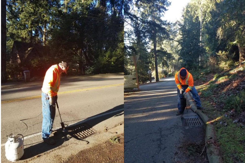
Catch basin & asphalt berm repair to assist in catching surface water sheet flow on 47 th Ave near NE 178 th St.
