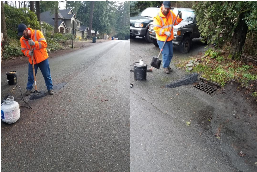
Pothole repair on 26 th Ave NE and additional surface water berm for directing the sheet flow to the catch basin.
